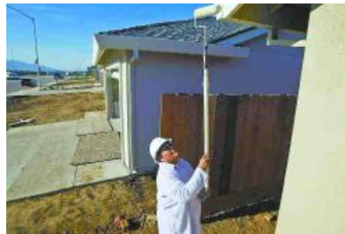
SCOTT MACDONALD/THE SALINAS CALIFORNIAN Dora Perez of Soledad, an instructional aide at San Vicente Elementary School, paints a house being built by CHISPA on Monday in Soledad. Her own home, which she and others helped build from the ground up, is a few doors down.
